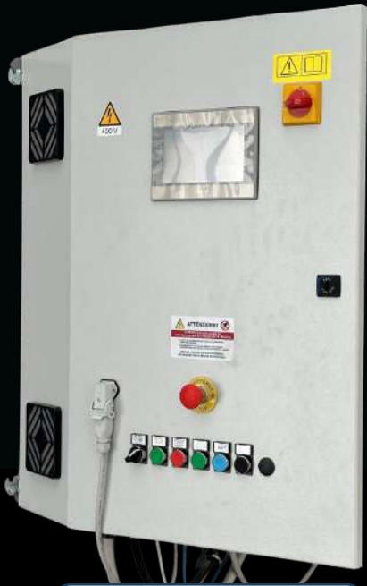
Panel de control
