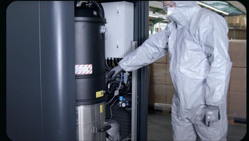
Easy access for maintenance
